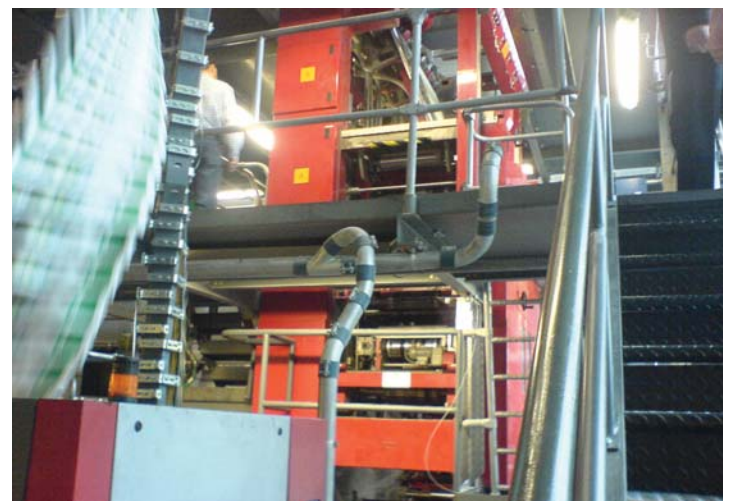
Dust extraction ducting integrates in plant operations
